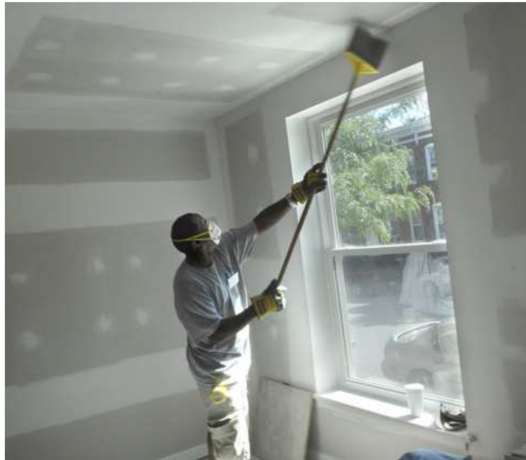
Donald Smith sweeps dust from sanded drywall during Sandtown Habitat for Humanity's "Summer Building Week." Over 20 years, the group has renovated 265 rowhouses. (Baltimore Sun photo by Jed Kirschbaum / June 25, 2009)
